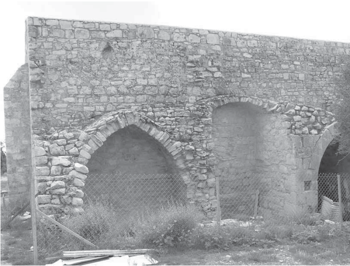
Fig. 62: Pano Polemidia, Karmiotissa, north wall with remains of conventual buildings [M. Olympios].
